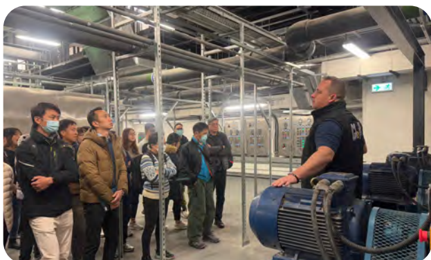
Trainees of the National Pool Plant Operator Certificate Course visited the plant room of the Tung Cheong Street Swimming Pool which is one of the most advanced pool plants in Hong Kong.
